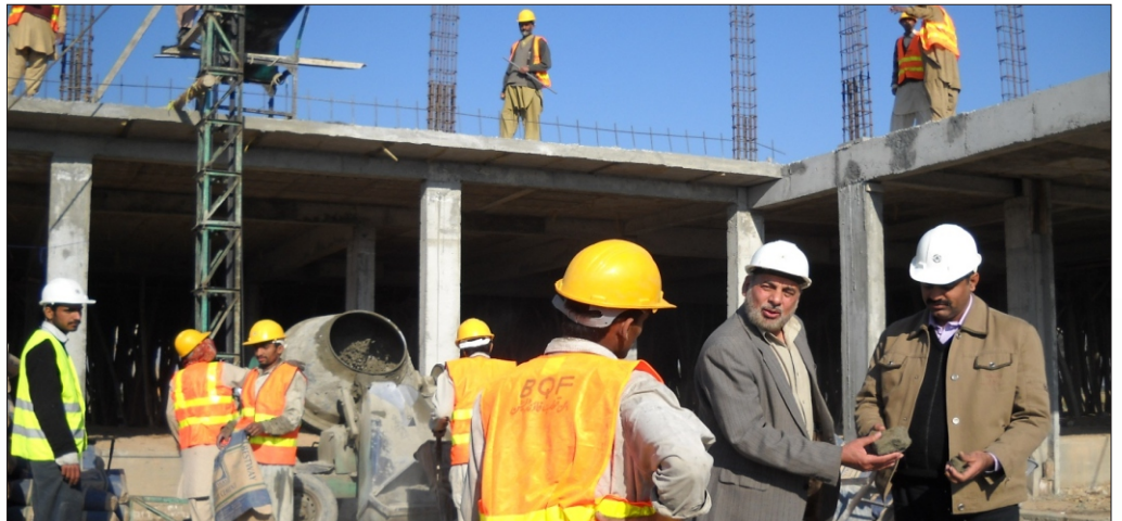
Brig (r) Dr. Riaz Ahmed Raja, CEO BNMH & Faisal Malik, Co-Founder and Director BQF at site, inspecting Quality of Material For First Roof.
