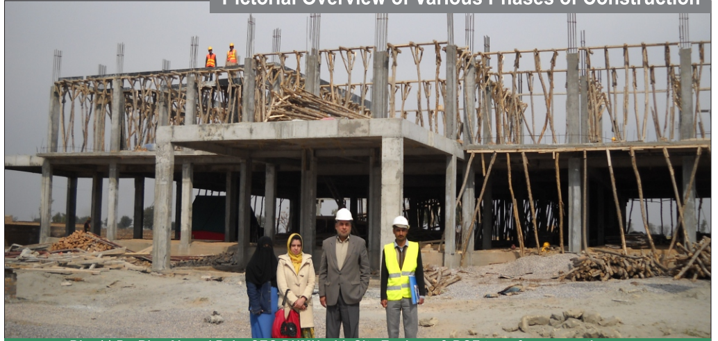
Brig (r) Dr. Riaz Ahmed Raja, CEO BNMH with Site Engineer & BQF team for preparation of 2nd roof on 17th Feb, 2012
